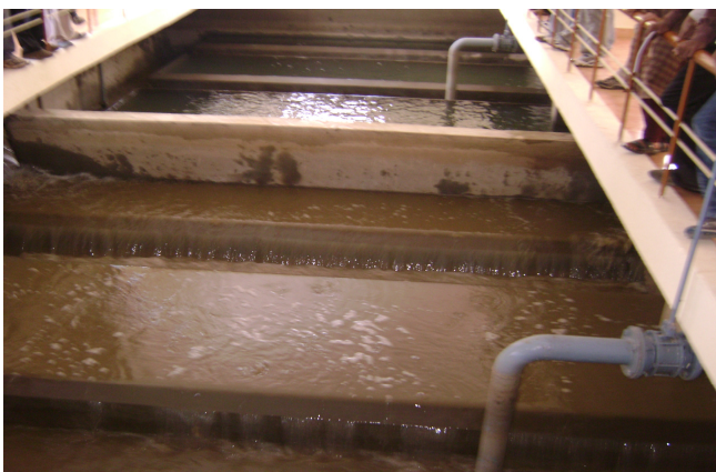
Backwashing of Sand Filter
