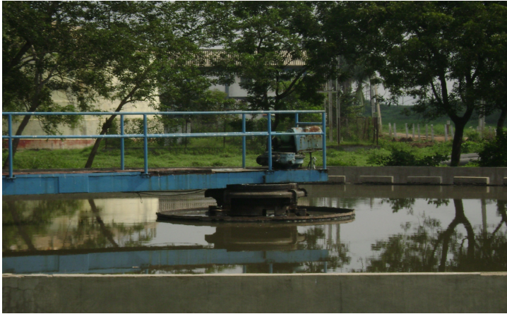
Primary Clarifier of STP
