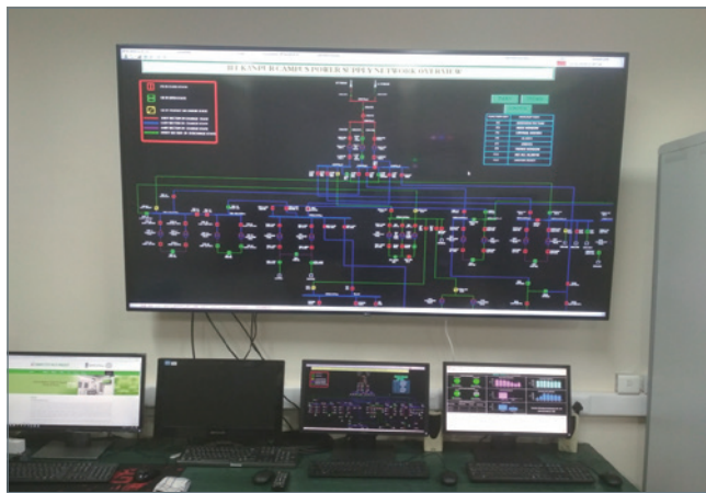
Figure 9-23. Monitoring and Control System at IIT Kanpur's Smart City Pilot project.
