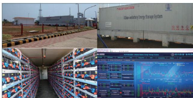
Figure 9-15. Grid scale Battery Energy Storage System at Puducherry
