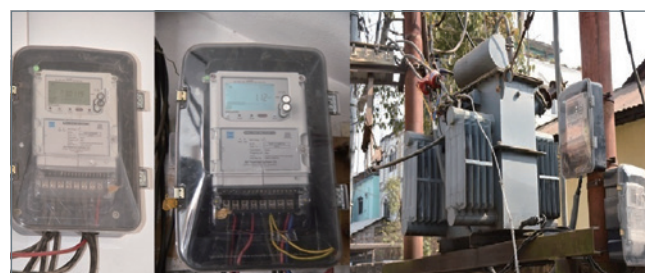
Figure 9-21. AMI Installed in the Distribution System
