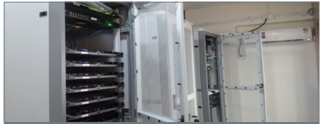
Figure 9-12. SG Control Centre (Servers) at Mysore
