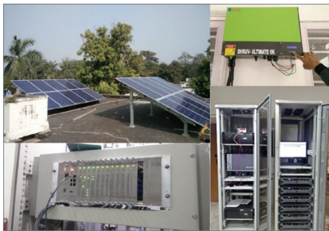
Figure 9-22. Deployment of Smart Grid Pilot Project at IIT Kanpur
