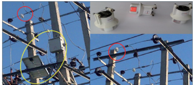
Figure 9-13. Communicable FPI Installations at Mysore
