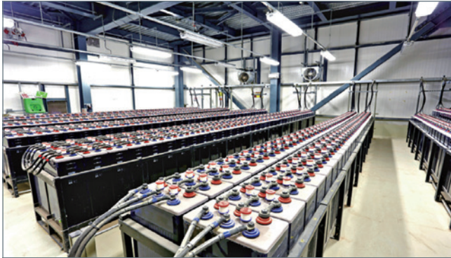
Figure 9-11. 10 MWh Battery Storage Bank
