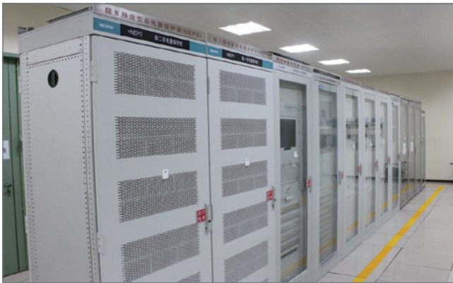
Figure 4-9. The Coordinated Control Station Of Three Gorges DCs
