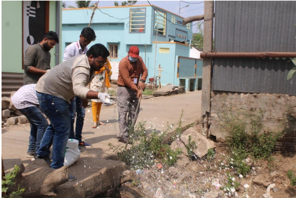
Clogged drainages were cleaned and Bleach powder is sprinkled in order to avoid bad smell
