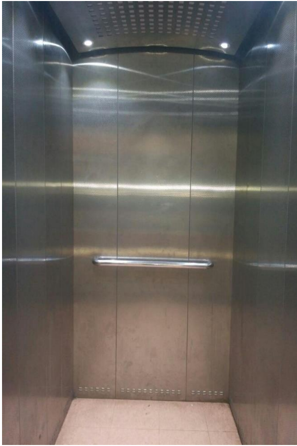
CENTRAL LIBRARY BLOCK LIFT RAILING FACILITY(SENSOR BASED LIFT DOORS)
